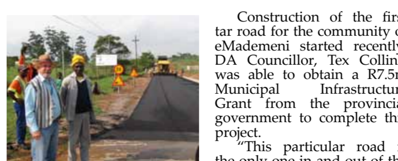
DA Cllr Tex Collins inspects the progress being made in the construction of the first tar road in eMademeni.
